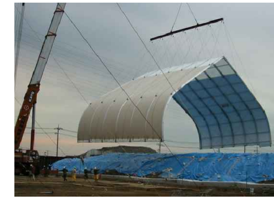
5 A1.1g SKATING RINK ROOF STRUCTURE REFERENCE PICTURE SCALE: N.T.S. SIMILAR DESIGN SCHEME ONLY
